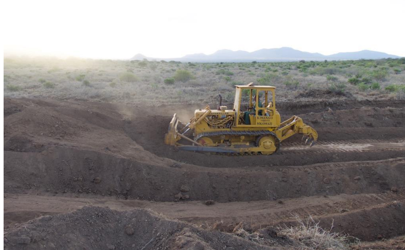
Bulldozer at work on the creation of a new water source in Mkomazi National Park for elephant herds and other wildlife
