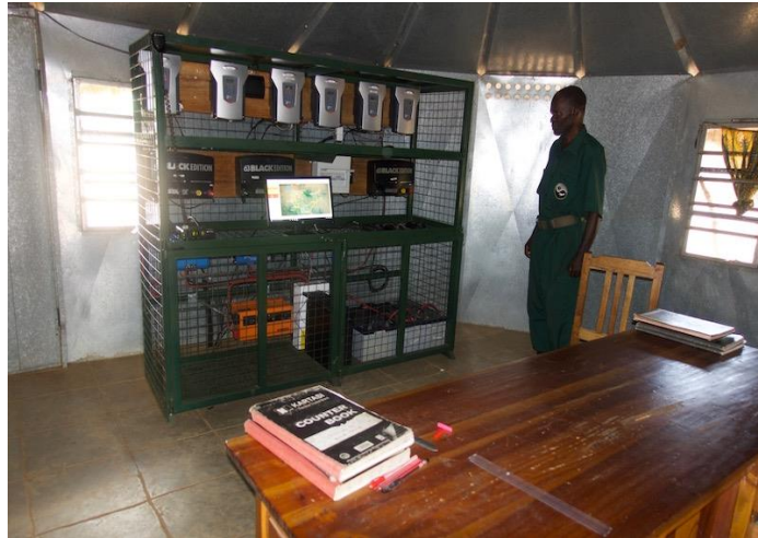
New energizers and alarms fitted
